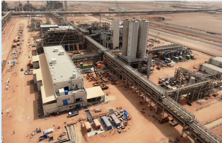
Borouge Ruwais Project, 2013
