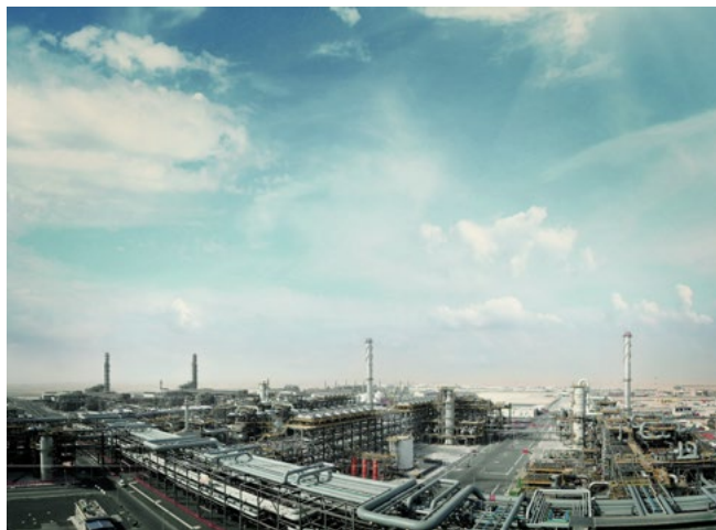
Habshan 5 - Gas Field Development Project - Sulphur Recovery Units & Acid Gas Removal Units, UAE, 2009 – 2013.
