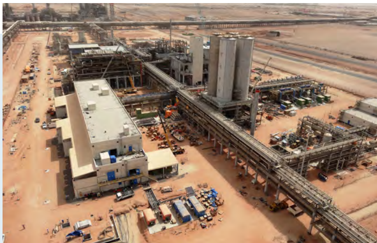
Borouge Ruwais Project, 2013
